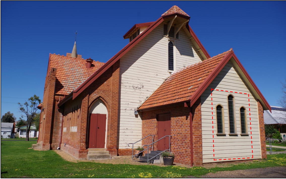
Figure 27: Temporary openings in two northern timber framed and clad walls. (Source: BT and MS)
