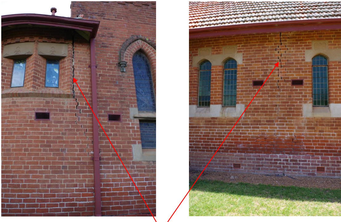
Figures 16 & 17: Substantial cracking to eastern wall of church. (Source: Michael Scott, Feb 23)
