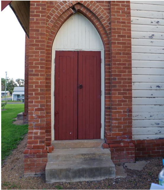
Figure 29: Concrete stairs to be removed, northern end of East Aisle. Note: conc. stairs outside Vestry are similar.
