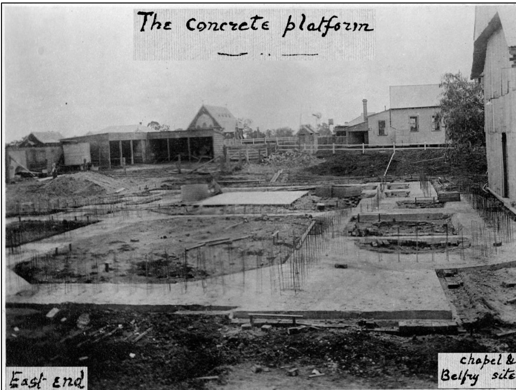
Figure 7: Shallow, reinforced concrete footings constructed in the 1920s (Source: St Ambrose archives)
