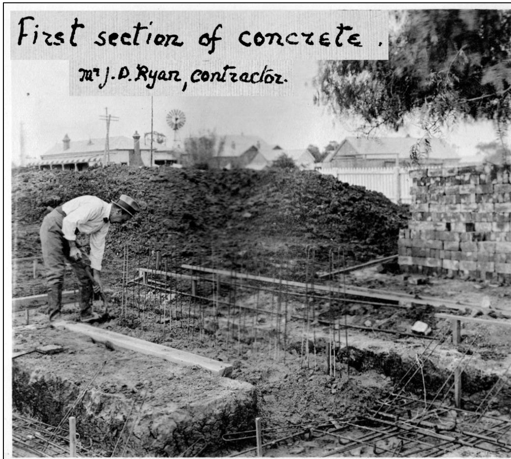
Figure 5: Shallow, reinforced concrete footings constructed in the 1920s (Source: St Ambrose archives)
