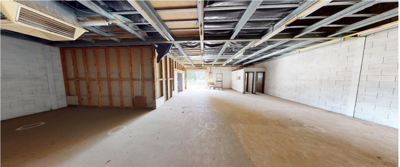
FIGURE 12. INTERIOR OF EXISTING BUILDING ON SUBJECT SITE, VIEW TO SOUTH-EAST TOWARD LOWER CASTLEREAGH ST
