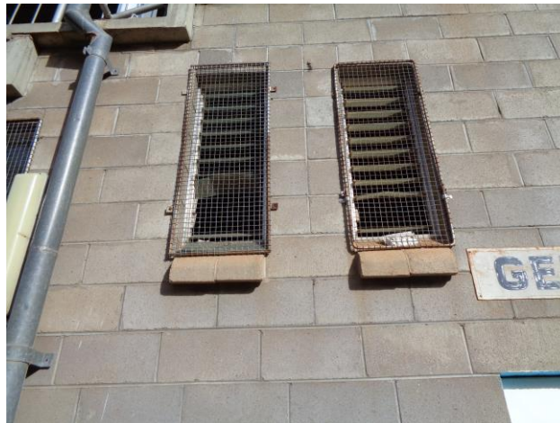
Figure 29 Broken, Cracked or Missing Louvres
