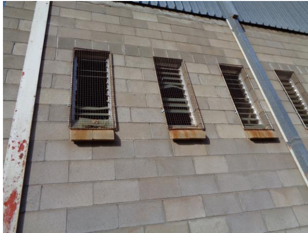
Figure 27 Broken, Cracked or Missing Louvres
