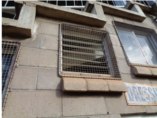
Figure 16 Broken, Cracked or Missing Louvres and glass window sashes to be replaced
