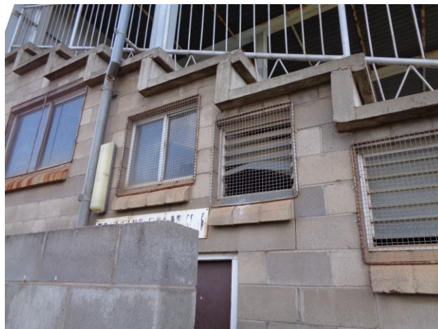
Figure 8 Broken, Cracked or Missing Louvres and glass window sashes to be replaced
