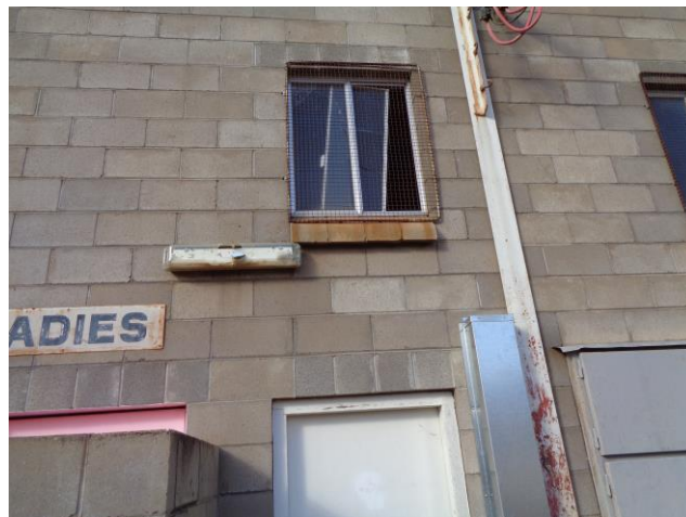
Figure 24 Cracked Glass Window Sash to be replaced, Replace External Light Fitting
